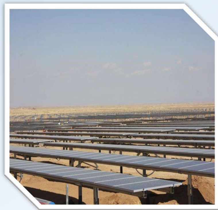
10 MW capacity grid-connected PV power plant (Isfahan Province, Iran)
