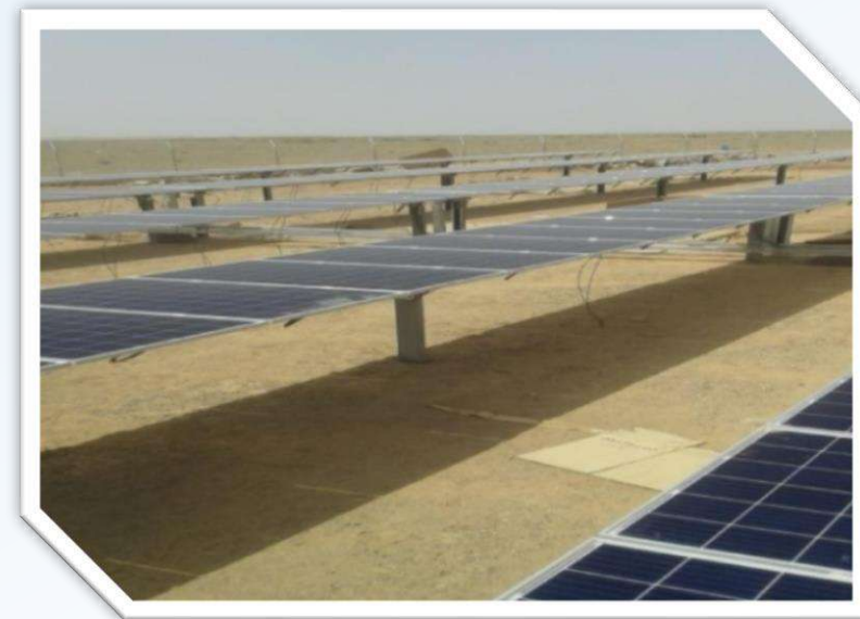
10 MW PV power plant (Qom Province, Iran)
