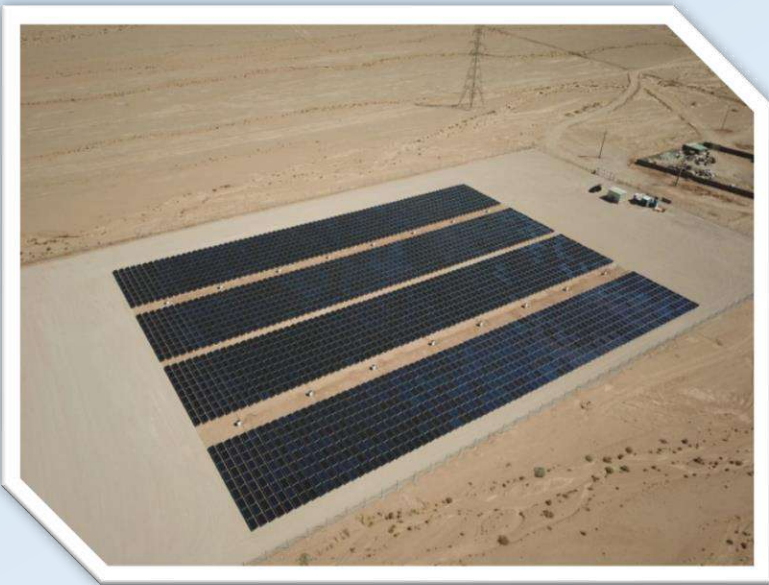
1 MW capacity grid-connected PV power plant (Razavi Khorasan, Iran)
